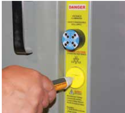
Fig. 9 Verifying proper operation of the NCVD
