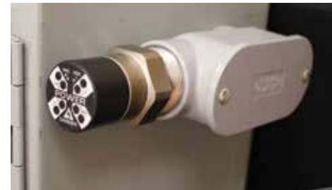
1 1/2 conduit vertical with R-3W
