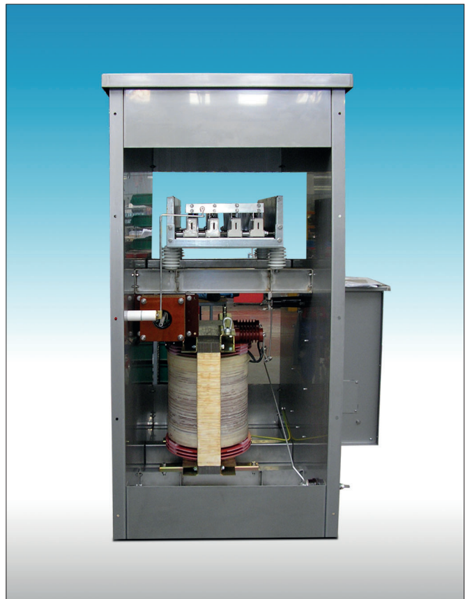
Single phase transformer with secondary resistor.
